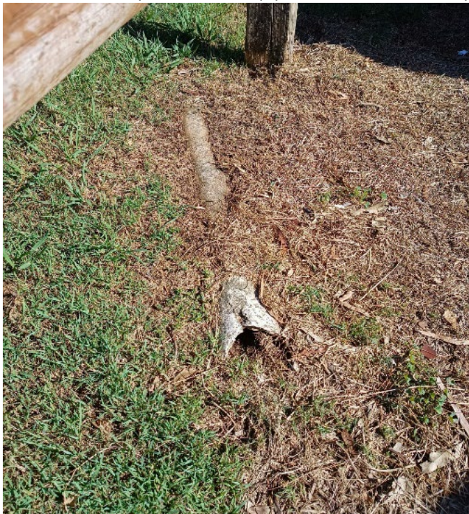
Figure 6-8. Exposed cement pipe
